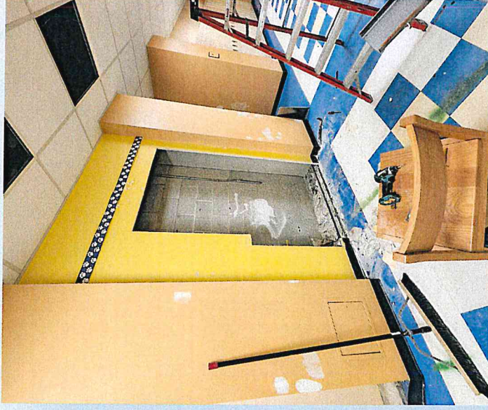
Hallway area: Removal of lockers, water bubblers, and opening the walls for access to the new bathroom doorways.
