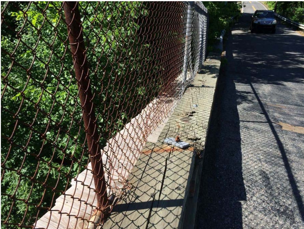
Photo 6: Curb area leaning into roadway; typical throughout both curbs.
