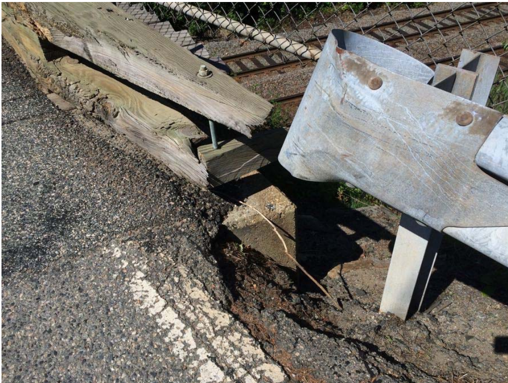
Photo 8: East approach, washout/settlement area at the north corner of the east abutment.
