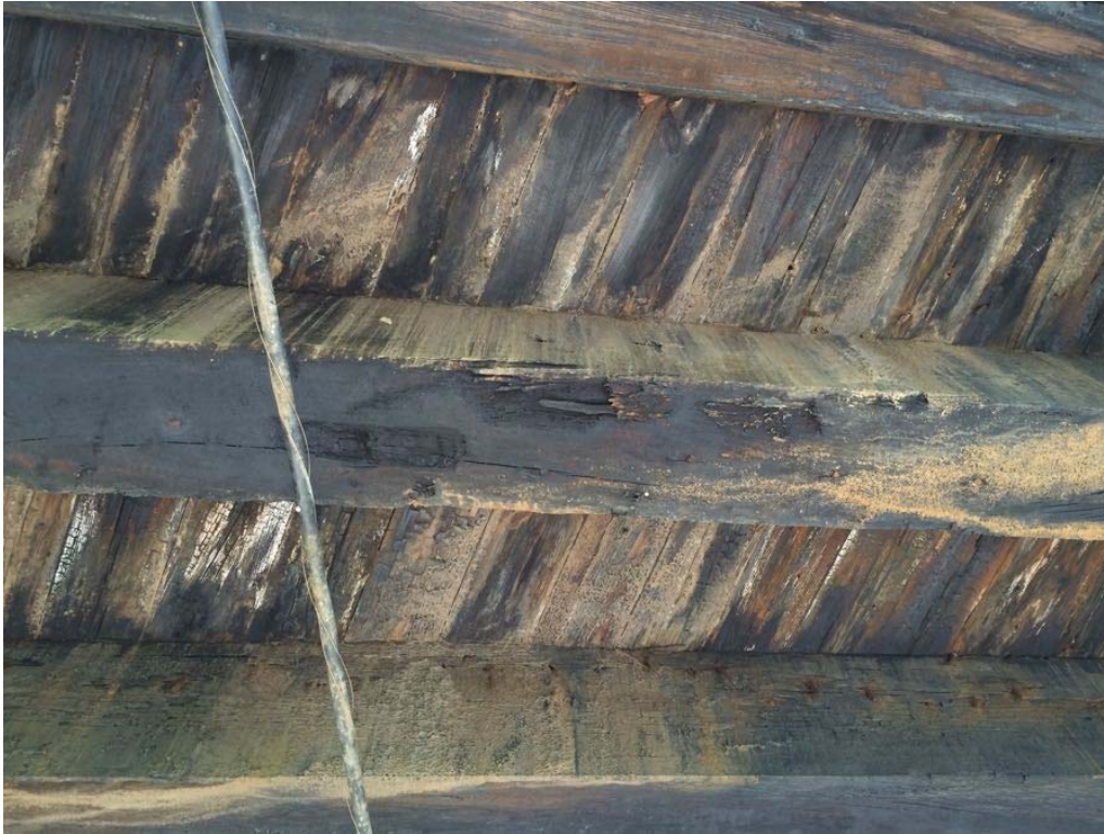
Photo 9: Typical areas of checking and splitting throughout all beams.
