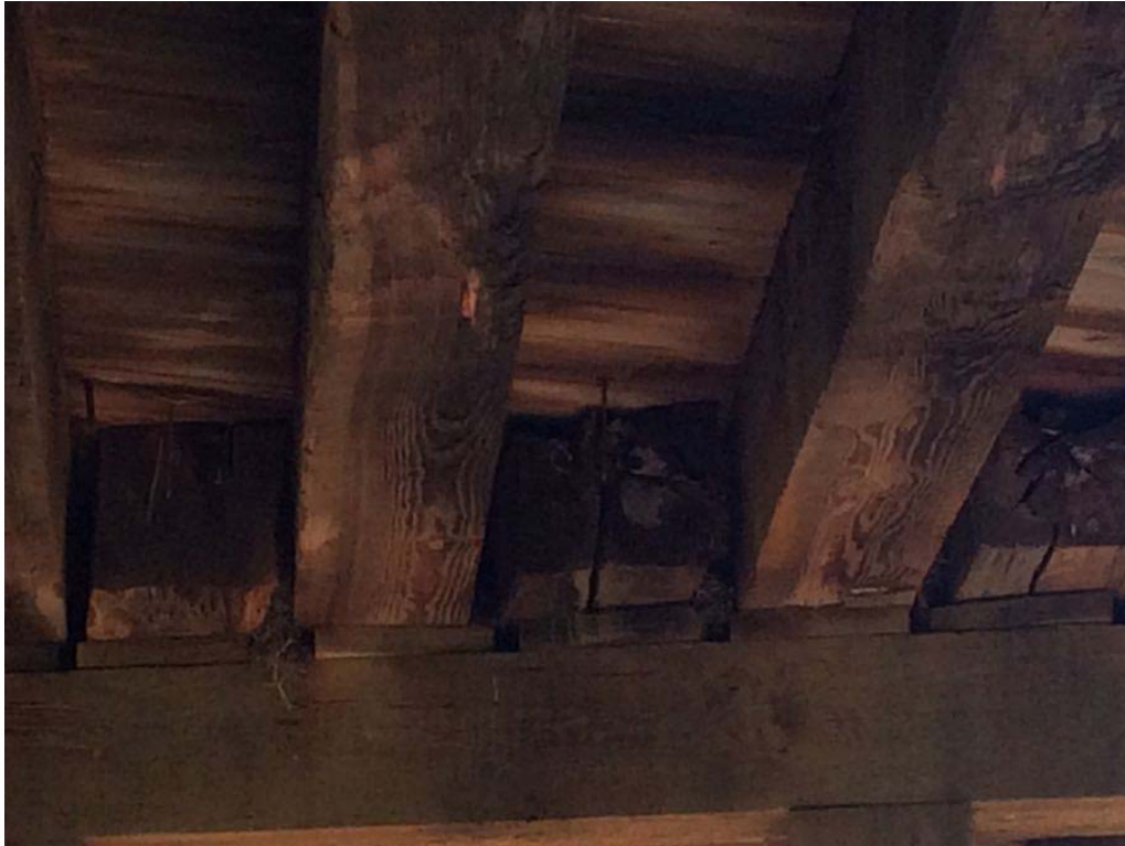
Photo 13: Span 3, west face of Beams 20 & 21, evidence of crippling and moderate splitting.
