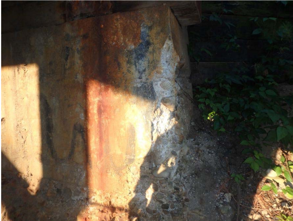
Photo 15: West breastwall, north end spalling.
