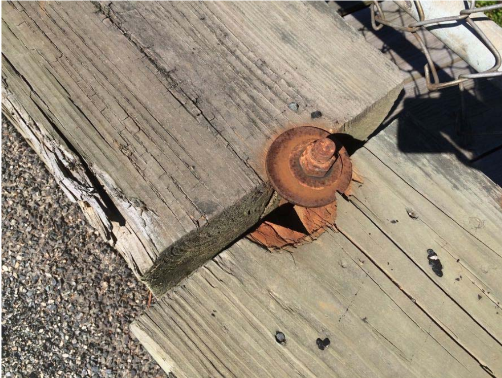
Photo 5: Typical broken connection throughout both curbs.
