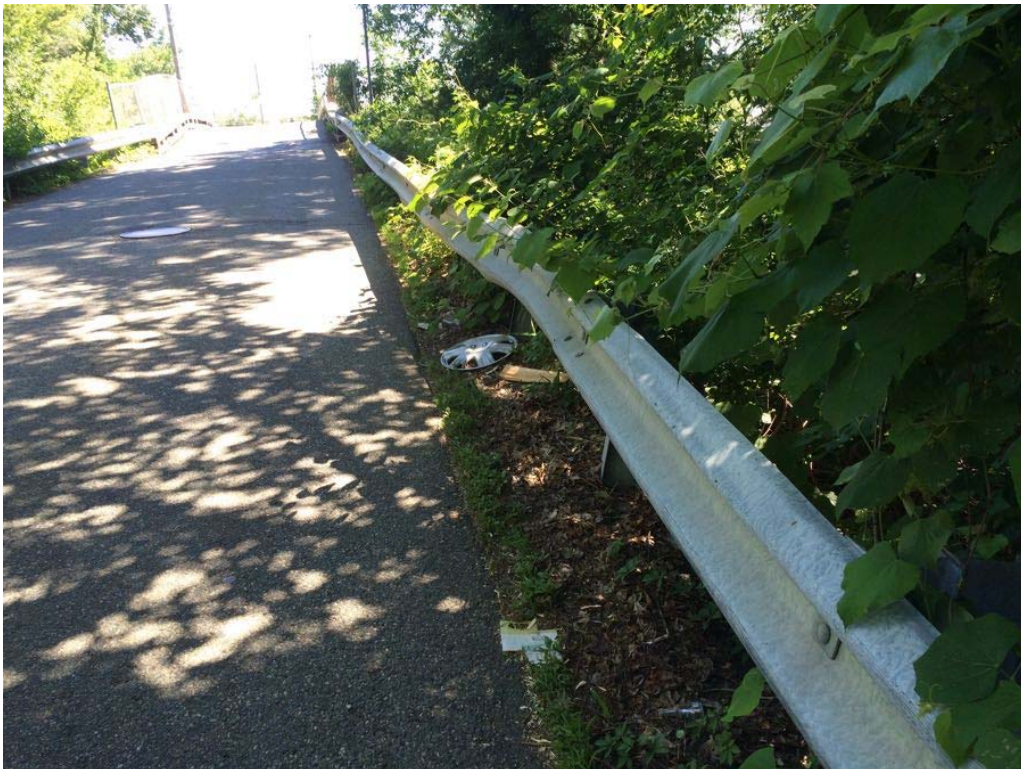
Photo 20: Southwest approach guardrail damage.
