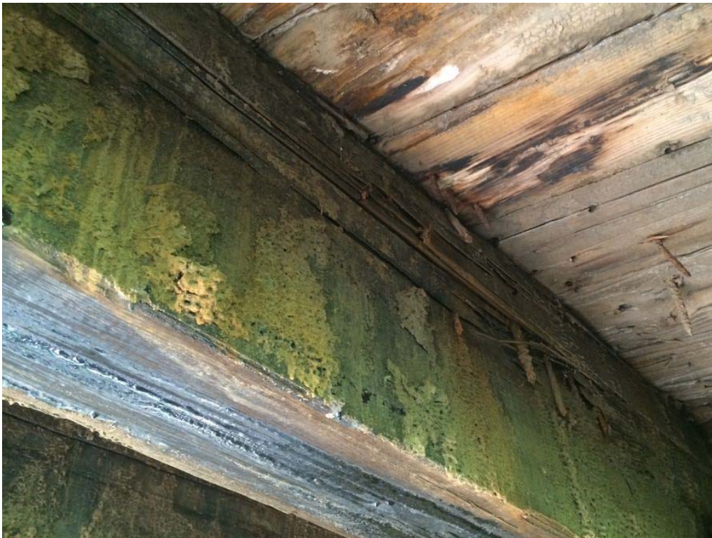
Photo 10: Span 1, typical areas of steel tie rods/nails popping out of both faces of all beams; typical splitting.
