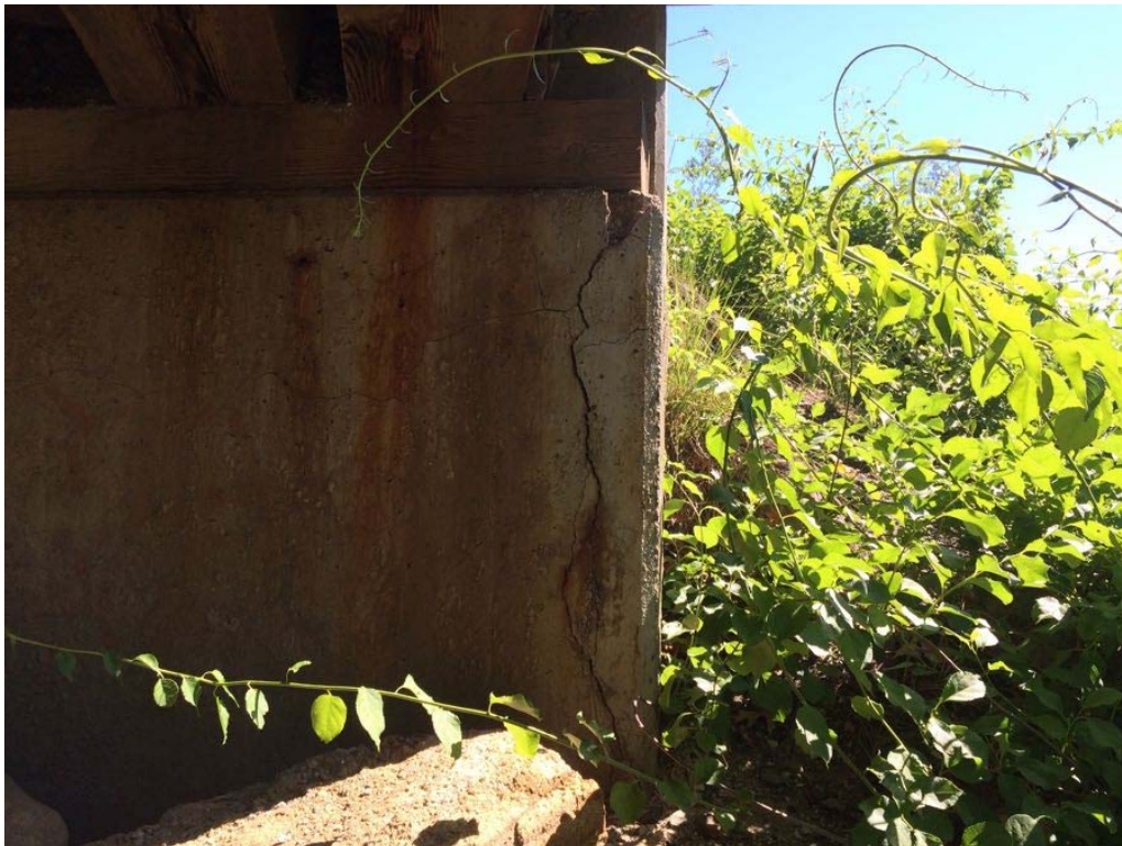
Photo 16: East breastwall, south end vertical crack.
