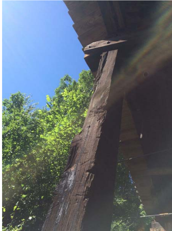
Photo 17: Pier 1, Column 1, typical rotting along the full height of the edges.
