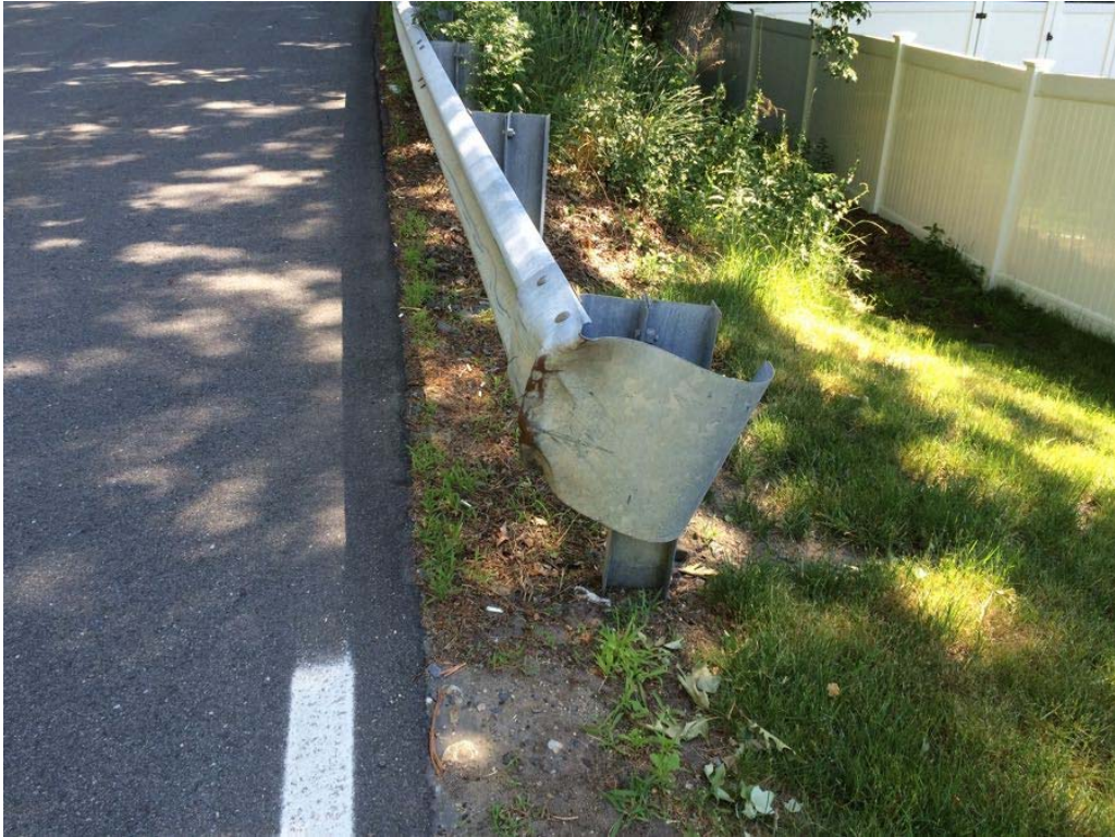
Photo 21: Southwest approach rail end damage.
