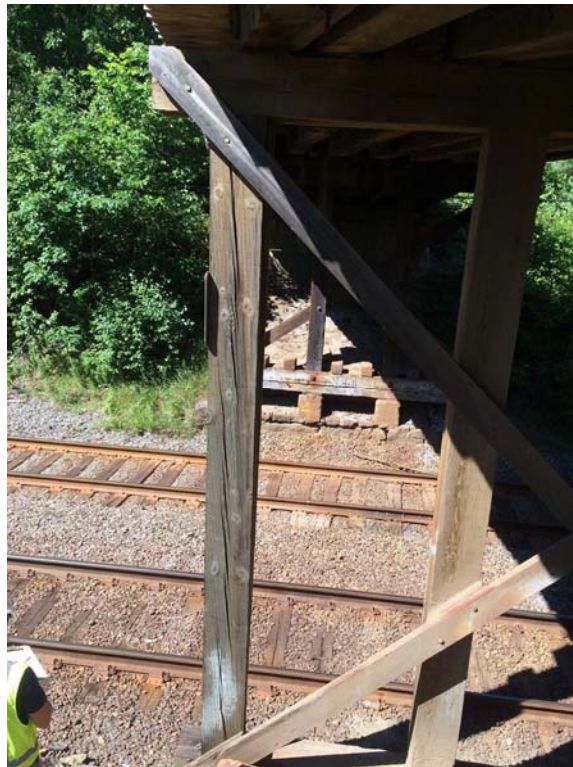
Photo 18: Pier 2, column 1, typical vertical splitting.
