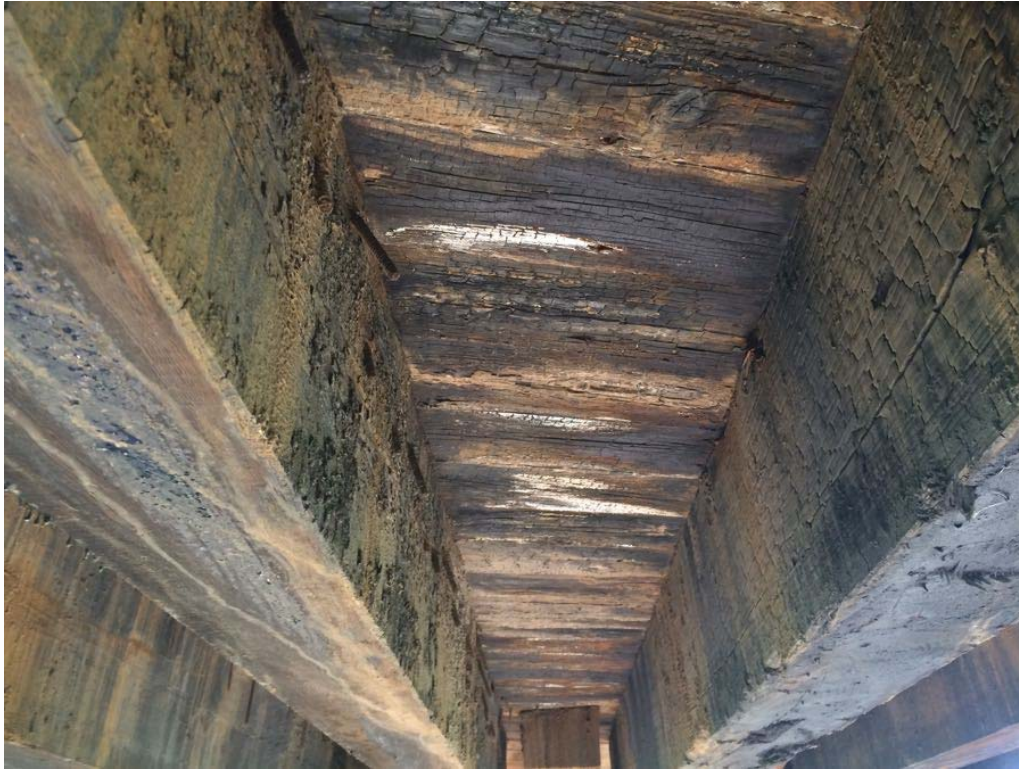
Photo 3: Typical rotting, checking, and efflorescence throughout the deck.
