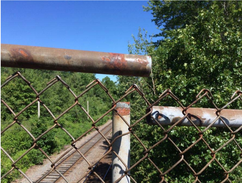
Photo 7: Typical broken fence connection; view of south fence near the west end.
