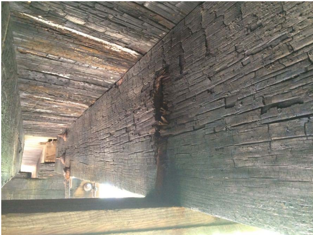
Photo 12: Span 3, typical view of random steel tie rod popping out of beam face.
