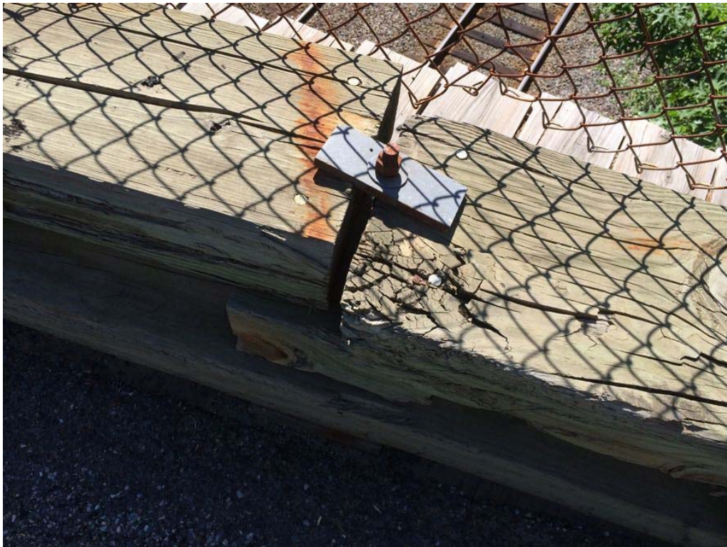
Photo 4: Typical timber curb deterioration and loose connection.
