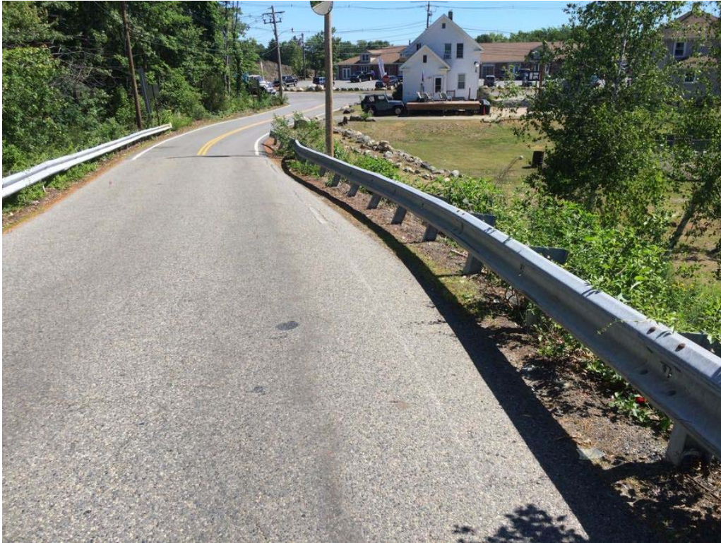
Photo 19: Southeast approach guardrail damage.
