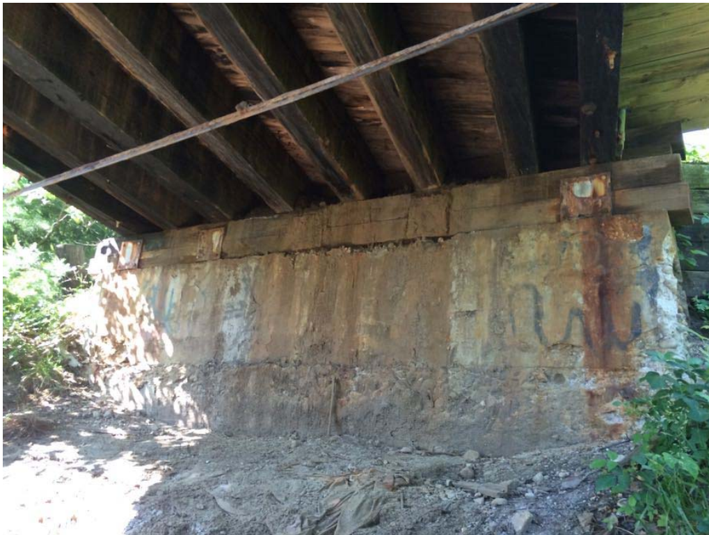
Photo 14: Typical scaling throughout both breastwalls; view of west breastwall.
