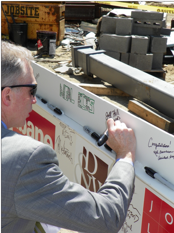
Town Manager Hull signs the final beam for the high school before it is hoisted into position at the Topping Off Ceremony in June
