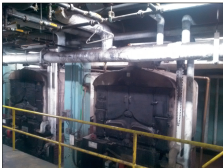
North Intermediate School Boilers
