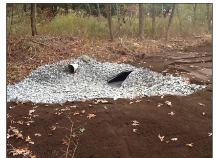
Drainage outfall for new drainage system
