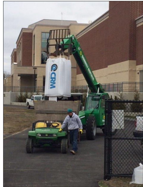
Bags of Crumb Rubber for Turf Field
