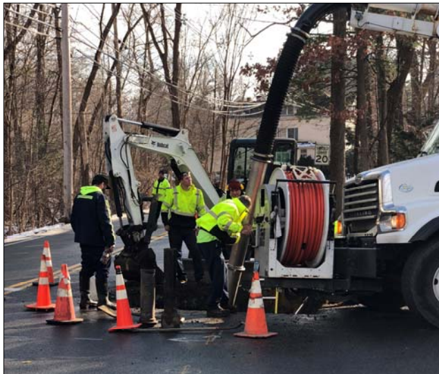
Water Main Break – Chestnut Street
