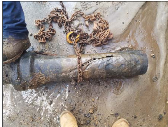
Broken Cast Iron Pipe – Grove Avenue/Main Street
