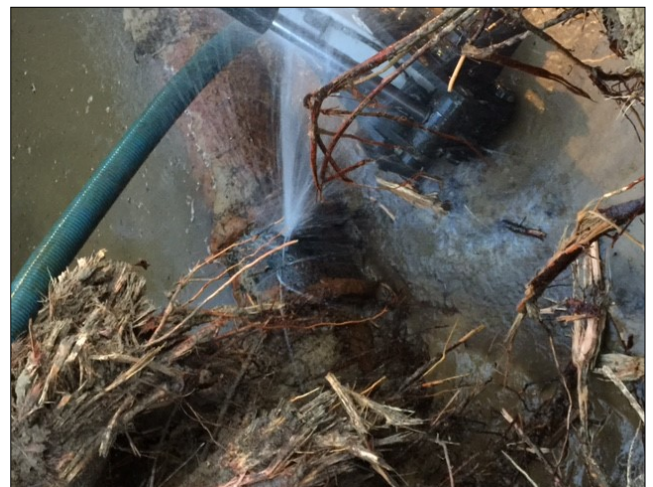
Water Main Break – Middlesex Avenue
