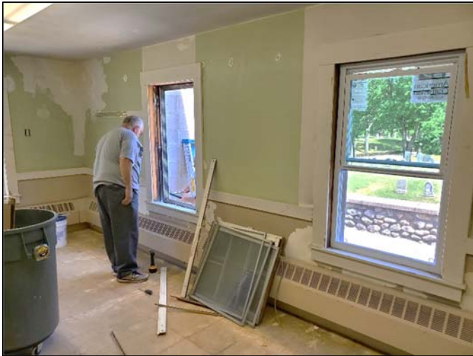
Former Town Hall/Arts Center Receives a Facelift in Preparation for Student Support Services New Offices
